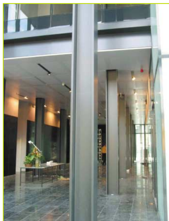
FIGURE 3 Banque Populaire with entrance hall and visible, unprotected steel columns in July 2003
