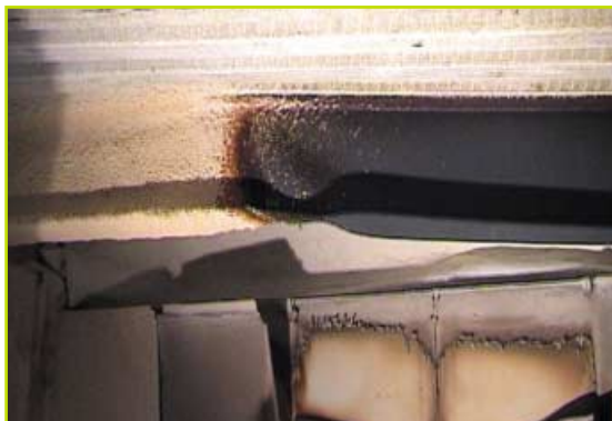
FIGURE 18: Plastic hinge in the unprotected beam cross-section close to the end of fire protection
