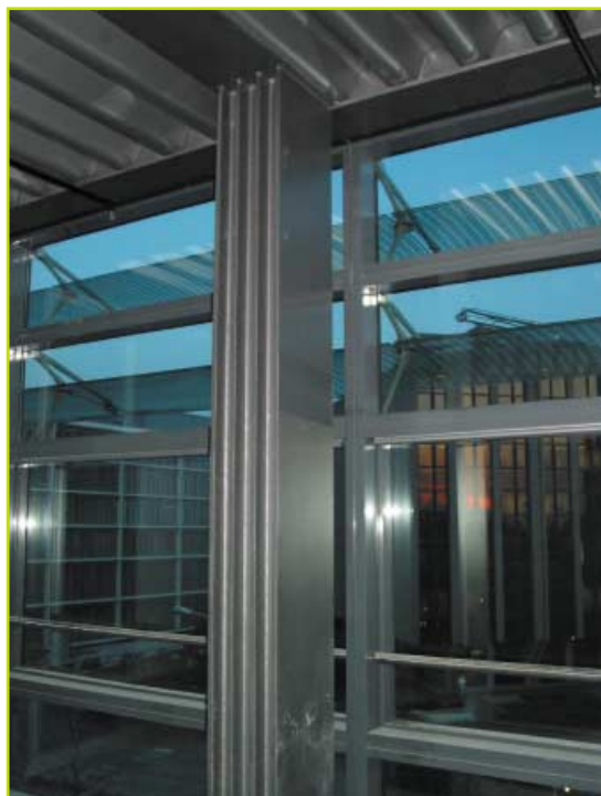
FIGURE 5 Chambre de Commerce with visible, unprotected steel columns supporting the composite beams.
