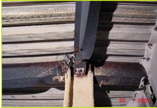
FIGURE 15: Local buckling of beam lower flange
