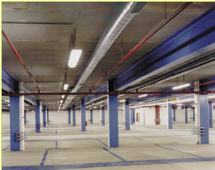
FIGURE 1 AUCHAN Phase II underground car park with unprotected 16,8 m long steel floor beams, in July 2000
