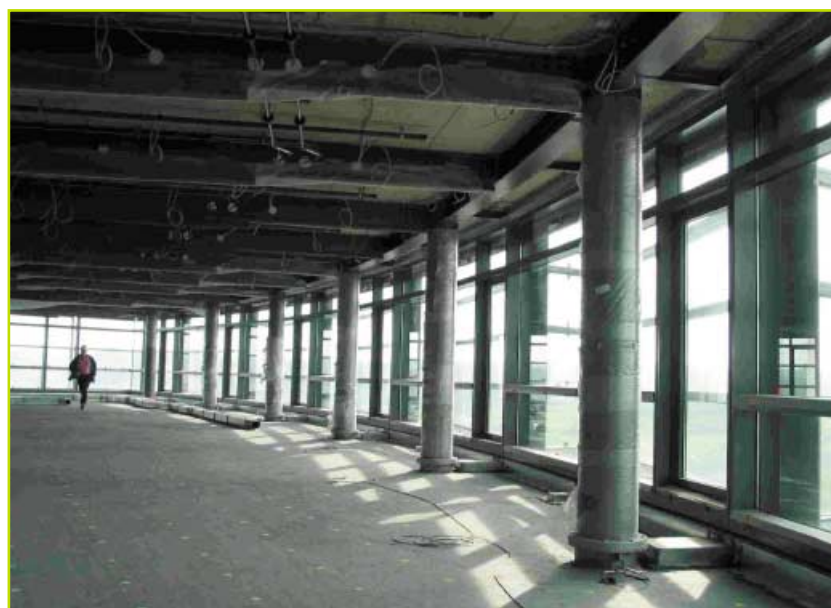
FIGURE 6 DEXIA-BIL building A; intermediate floor level with visible, unprotected composite circular columns supporting the composite beams
