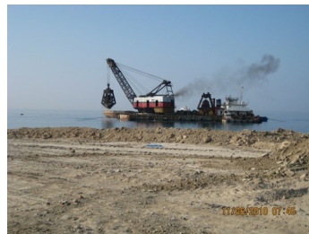
Figure 5 – Construction Stages 1, 2 and 3 – Reclamation for working space and protection from sea waves
