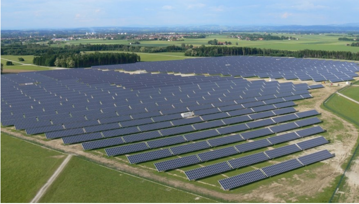
Fig. 3. A terrestrial type solar power plant
