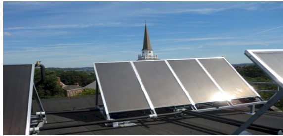
“The curtain-wall-type collectors installed in regular racks; the rooftop installation at Chatham University in Pittsburgh”
